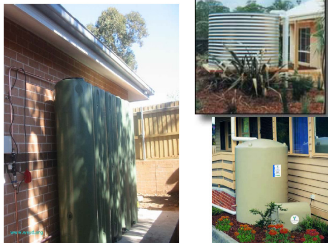
Figure 2.5 Water storage tanks, Australia
