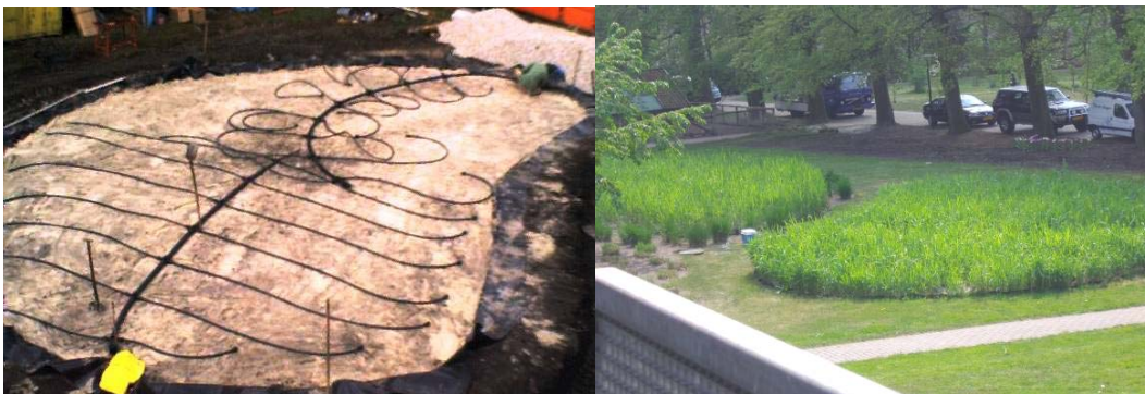
Figure 3: (i) CW during construction with distribution network and (ii) during the operation.
